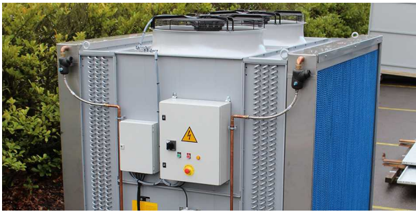
Waterfeed assembly connected to city water connection with flexible pipe
