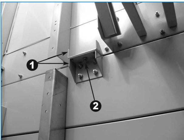
Plenum section installed on lower section
