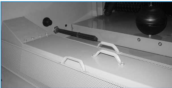
Cold water basin and basin strainer
