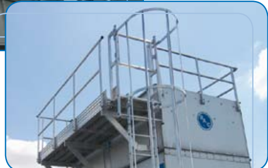
Access Ladder, Safety Cage, Platform and Handrailing
