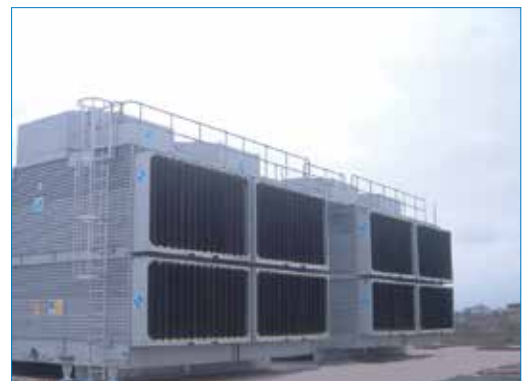
Figure 11: Intake and discharge sound attenuation on a BAC Axial Fan Open Cooling Tower
